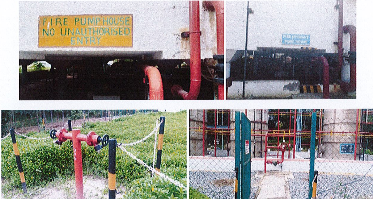
Fig. Firefighting systems
