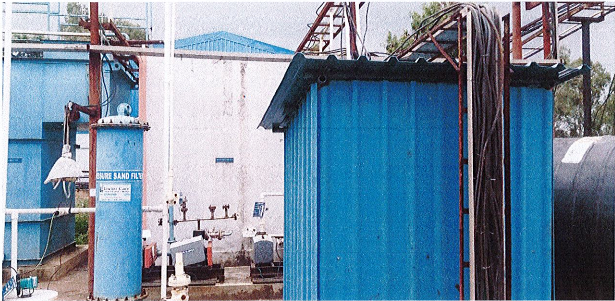
Fig. Sewage Treatment Plant (STP)
